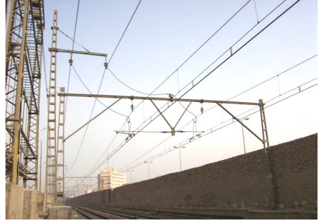
Fig. 4. DC Substation Supplies Line 1 and Line 2
